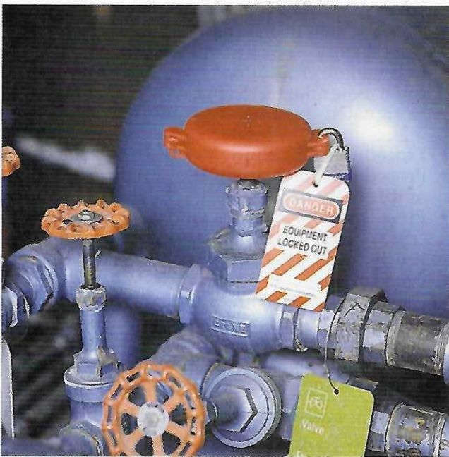
Figure 46 Placing a lockout/tagout device.
